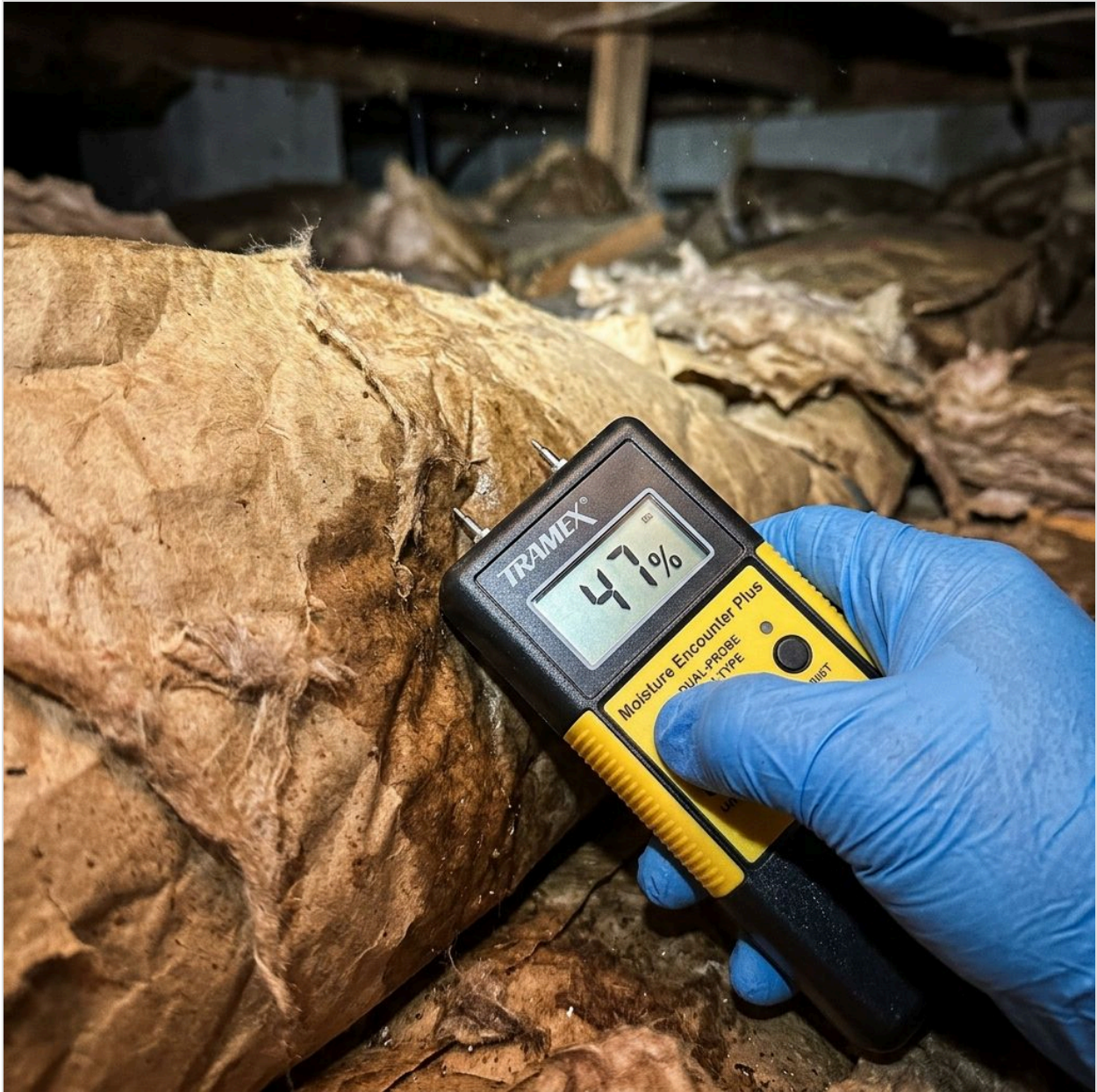
Pin moisture reading of 47% WME on degraded kraft-faced insulation at the south crawlspace rim joist. Reading exceeds the instrument's reliable upper range. Insulation shows significant staining and deterioration consistent with prolonged wetting.
