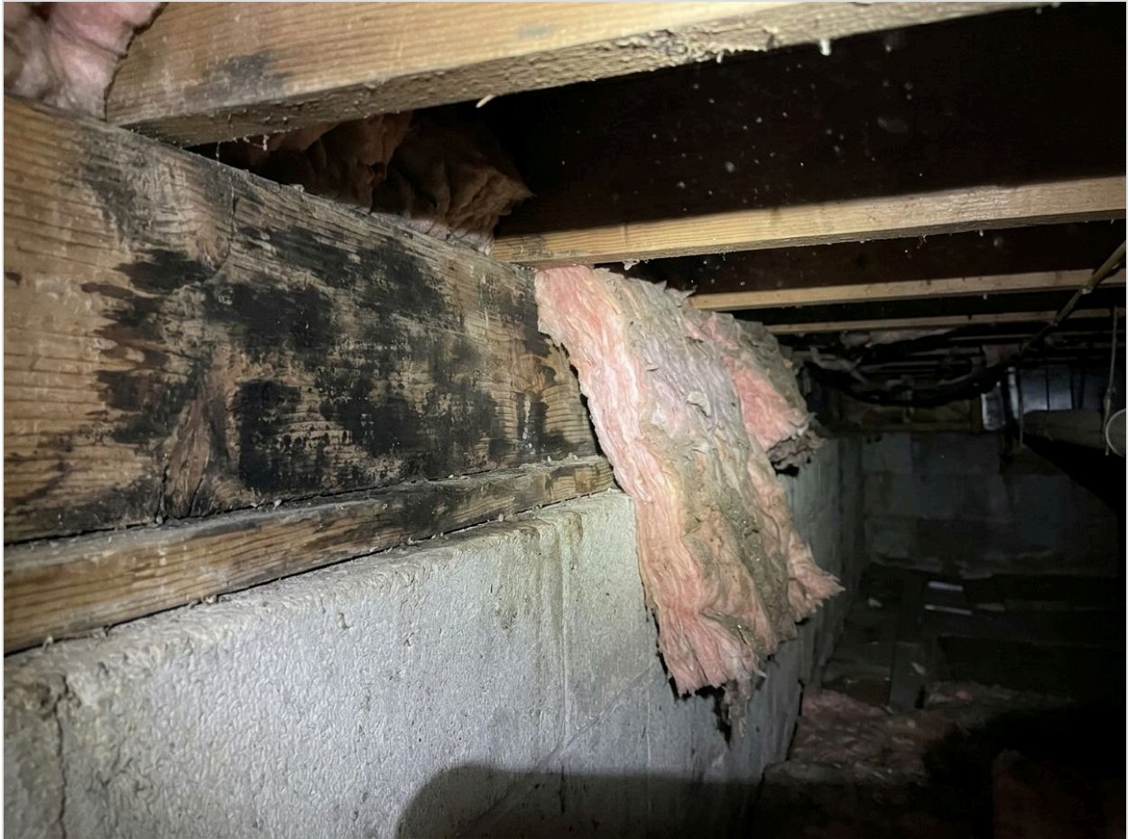
Extensive black and brown fungal discoloration on the sill plate and band joist at the south rim, consistent with active mold colonization. Displaced fiberglass batt insulation and concrete block foundation wall visible. Conditions consistent with IICRC S520-2024 Condition 3.
