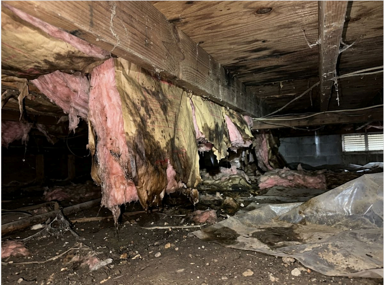
Fallen and sagging fiberglass batt insulation with dark brown to black fungal growth on kraft paper facing and subfloor decking. Active moisture dripping observed. Partial vapor barrier present on north floor only. Condition 3 per IICRC S520-2024.
