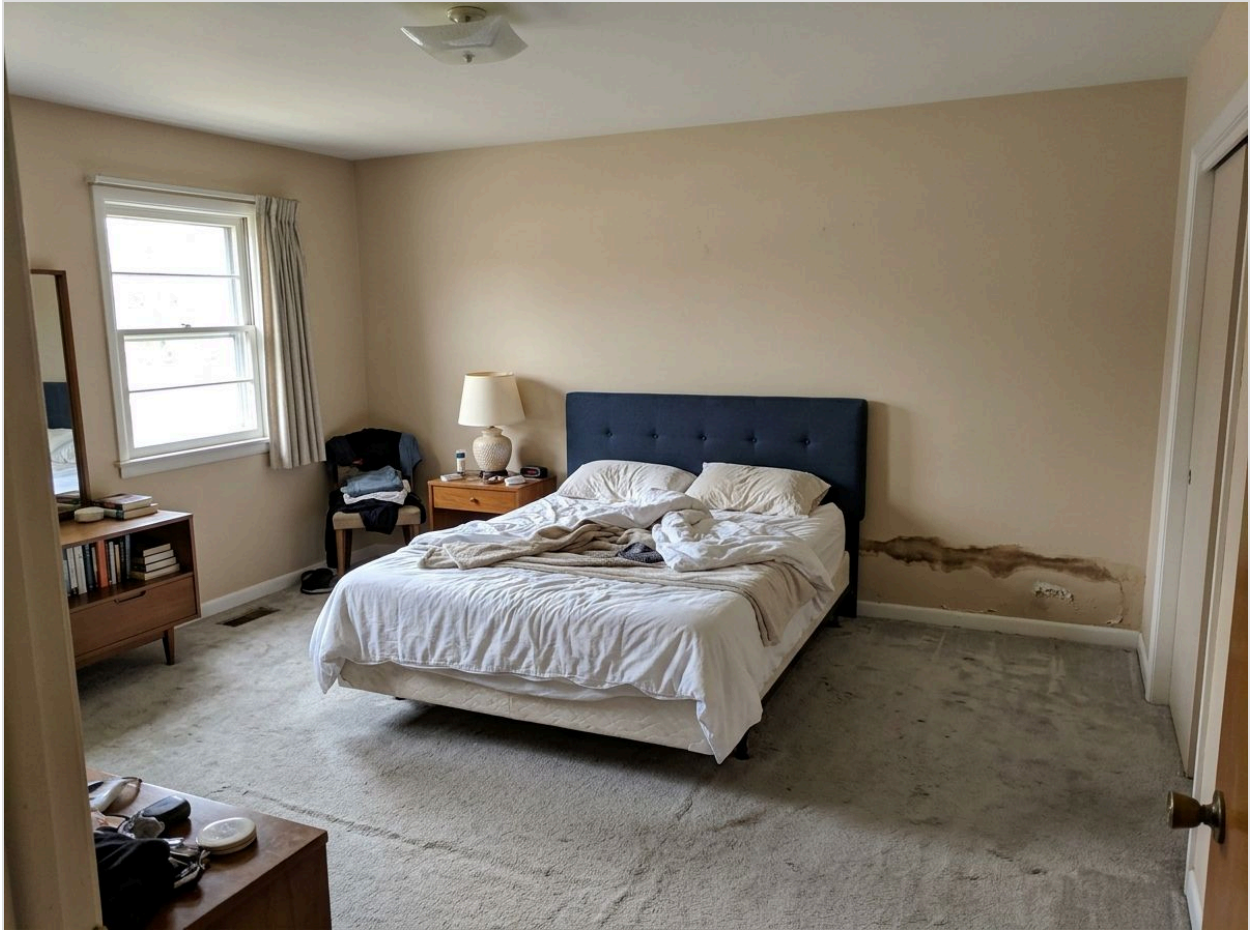
Brown water staining on the lower east wall, extending approximately 3 to 4 feet wide and 12 to 18 inches above the baseboard. Tideline demarcation and carpet discoloration consistent with chronic moisture intrusion at the wall base.
