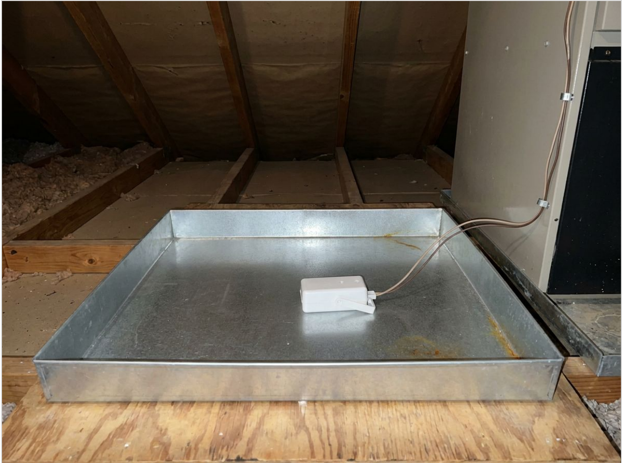
Secondary condensate drain pan beneath the attic air handler, showing float switch installed and wired to the unit. Rust-orange staining on the pan floor indicates prior water accumulation; pan is dry at the time of this visit.
