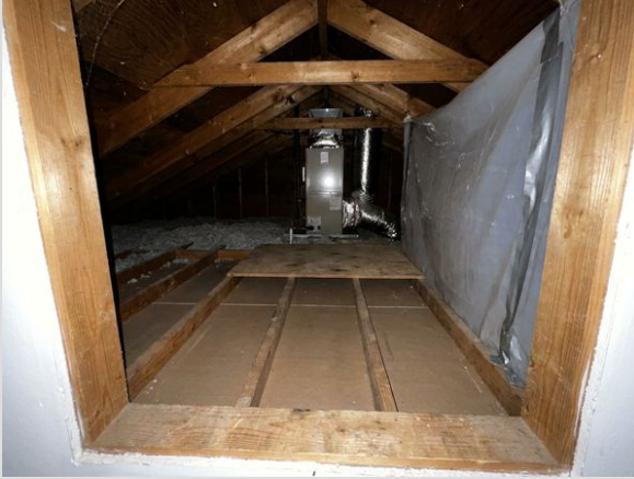
Attic — view from the scuttle after removal of the affected insulation
