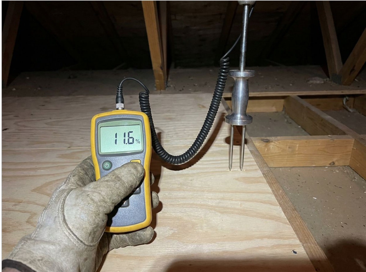
Pin-type moisture meter probe inserted into platform decking at the NE corner of the secondary pan footprint, reading 11.6% MC, below the drying goal of 13.4% MC.
