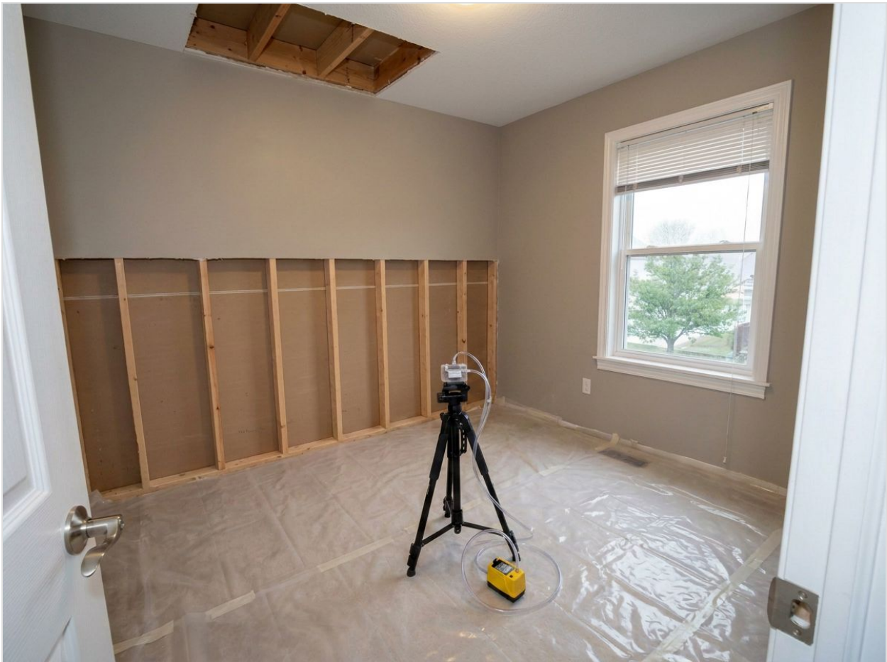
Bedroom 3 interior showing the post-remediation air sampling setup at center. West wall opened to the framing across the lower portion, ceiling section removed above the platform footprint. No visible mold growth or active water staining on exposed framing or remaining surfaces. Air sampling pump and spore-trap cassette on tripod visible at center.
