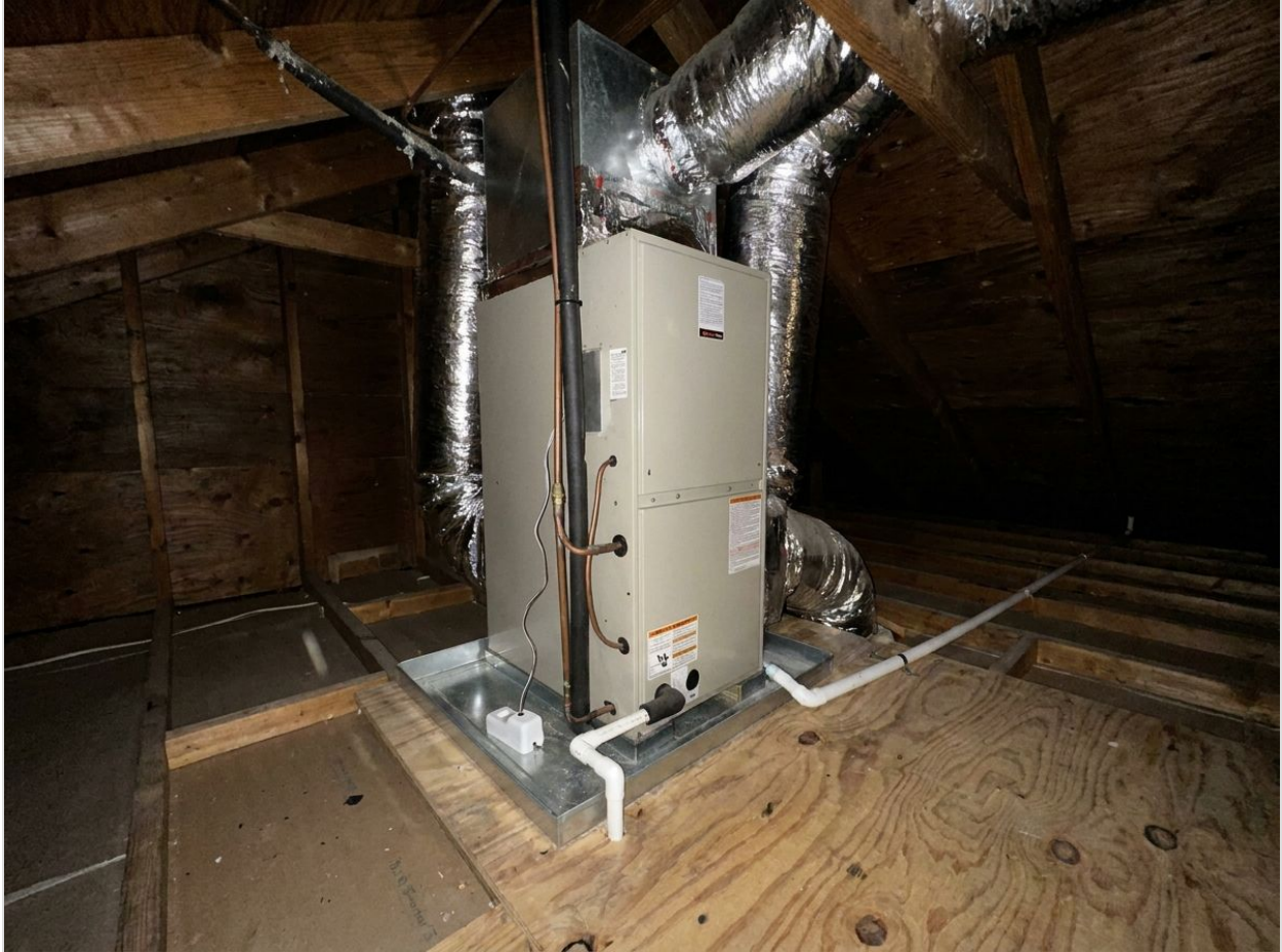
Attic air handler unit on the equipment platform, showing the galvanized secondary pan, PVC condensate drain lines, and refrigerant line set. No visible mold growth or active water staining observed.
