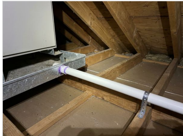
Attic — secondary pan drain line repiped to a termination
