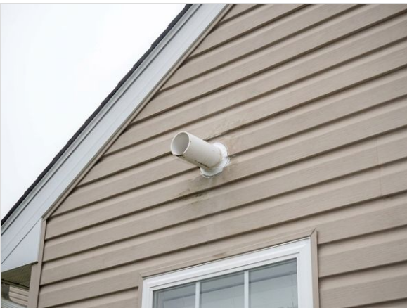
Exterior — new secondary condensate discharge termination
