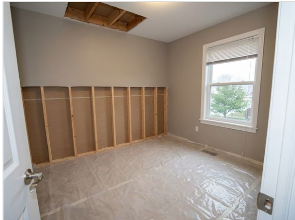
Bedroom 3 — affected materials removed, framing and wall cavity exposed
